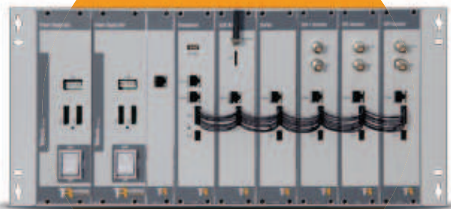
EXTERNAL ALARM MONITORING AND EQUIPMENT CONTROL
